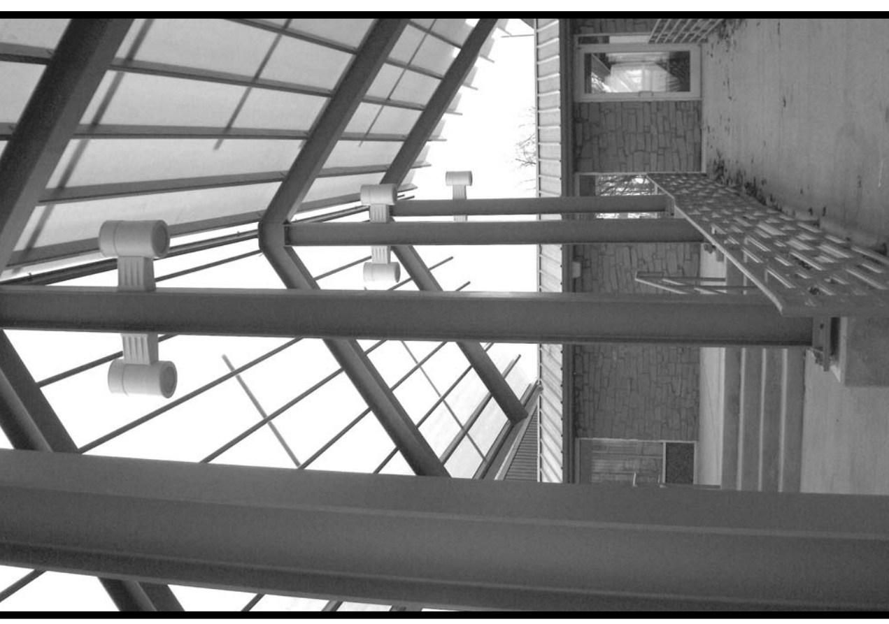
In January Stone Belt finished the "Safety Project" a new circular driveway and covered entrance on the North side of its 10th Street building in Bloomington. To learn more and view pictures from the construction see Page 4.
