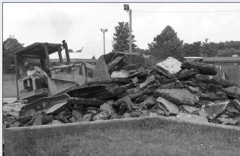
Phase one of the Safety Project involved tearing up old concrete that was in the area. A bulldozer assisted in this task.
