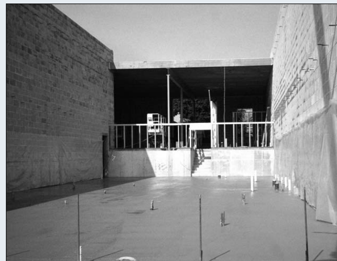
Concrete walls and floors have been erected. A stairway connects the addition's two floors. Next the roof will be added.
