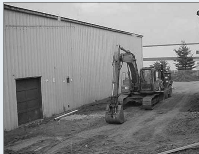
The corridor between the workshop and warehouse (left) was demolished to make way for the addition.
