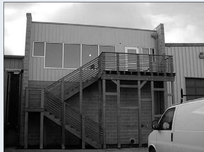
A view of the completed addition from the outside between the workshop (left) and the warehouse (right). The room above will be used for conferences and training.
