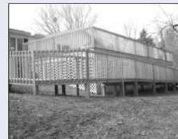
View of the new deck from the back of Maxwell House. The new deck measures 30x18. There are also two long ramps to lead residents into the yard.
